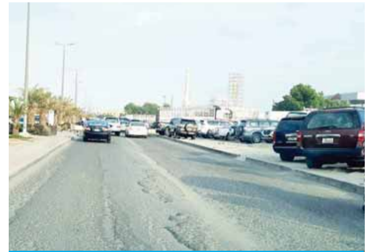
KUWAIT: This December 31, 2020 file photo shows a damaged road near the Friday Market. — Photo by Fouad Al-Shaikh
