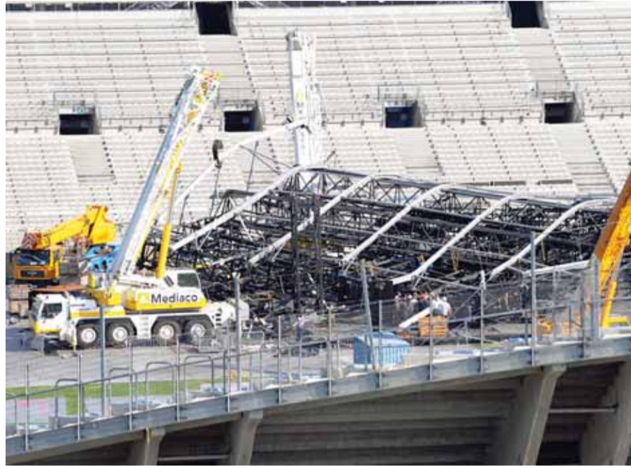
This file photo taken shows the Marseille's Velodrome Stadium after the collapse of a stage set up for a Madonna concert in which two stage hands died. — AFP
