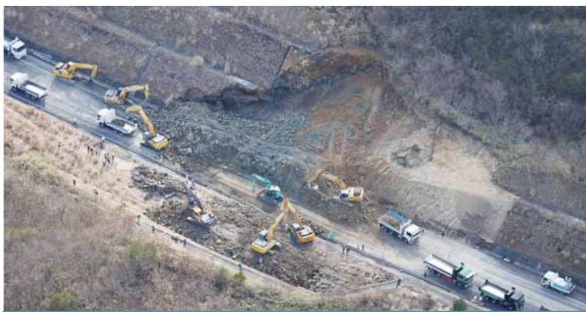
SOMA, Japan: This aerial picture taken from a Jiji Press chartered aircraft shows the landslide site on the Joban Expressway in Soma, Fukushima prefecture yesterday after a 7.3-magnitude earthquake struck off Japan's east coast. — AFP
