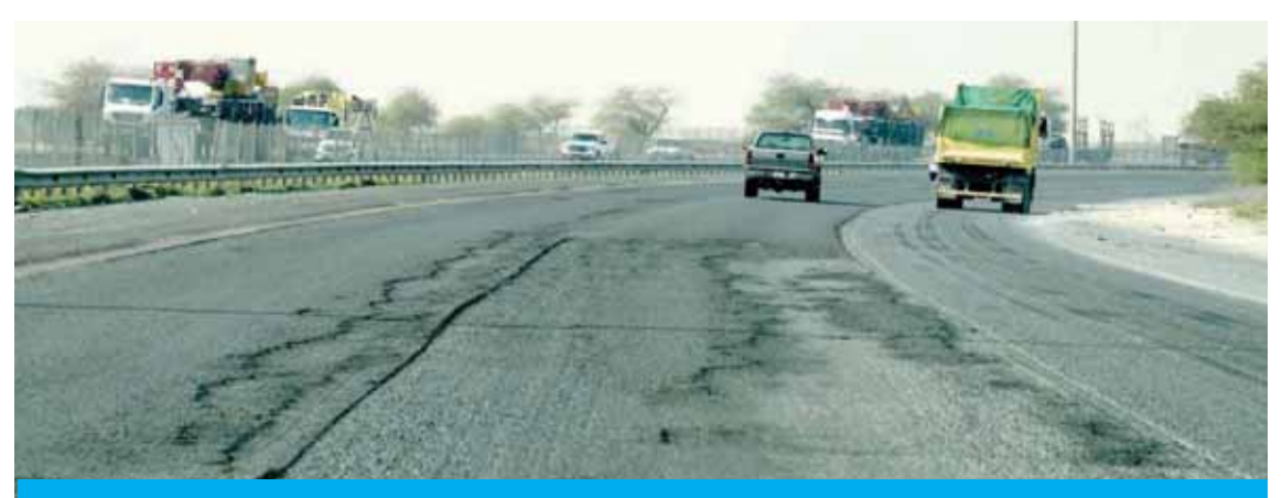
KUWAIT: A combination of photos showing a heavily damaged section of the Seventh Ring Road yesterday. — Photos by Fouad Al-Shaikh
