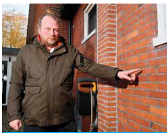
GARRELSWEER, Netherlands: Dutch resident Daan Schoolland, 41, shows the damage to his home two weeks after an earthquake measuring 3.2 on the Richter scale struck in Garelswaer, Groningen. —AFP
