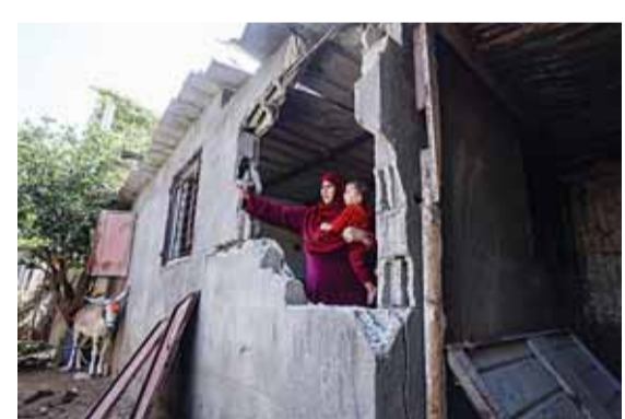
BEIT HANUN, Palestinian Territories: A Palestinian woman inspects the damage at her house following Zionist bombing in Beit Hanoun in the northern Gaza Strip yesterday. —CAFP
