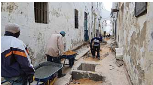
Laborers work on an infrastructure rehabilitation project in an alley of the Libyan capital Tripoli's Old City.
