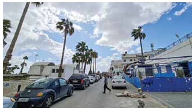
A man crosses a street in the Libyan capital Tripoli's Old City, amid ongoing infrastructure rehabilitation work.
