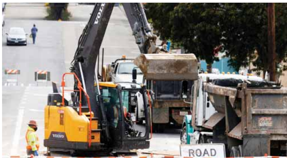
SAN FRANCISCO: Workers operate an excavator as they make infrastructure repairs on Wednesday in San Francisco, California. President Biden last week unveiled a $2 trillion jobs and infrastructure plan paid for in part by an increase in the domestic corporate tax rate, and by sweeping up corporate profits stashed overseas.—AFP
