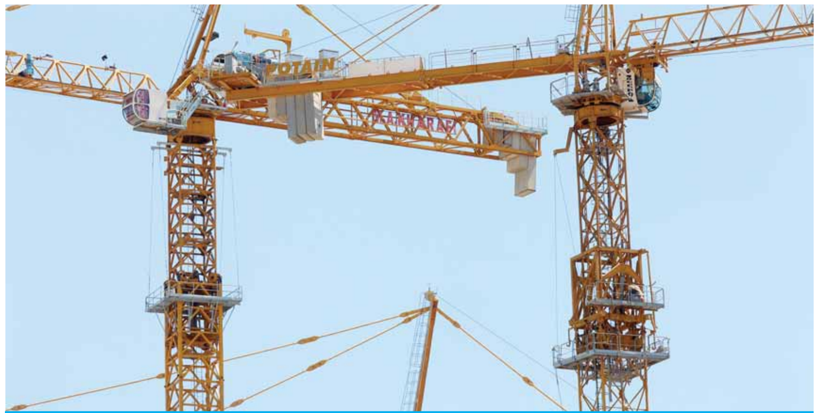
KUWAIT: Tower cranes seen at a major construction site in Kuwait City. — Photo by Yasser Al-Zayyat
