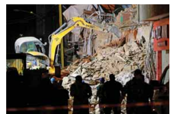
BEIRUT: Rescue workers dig through the rubble of a building in the Lebanese capital's Gemmayze area. — AFP
