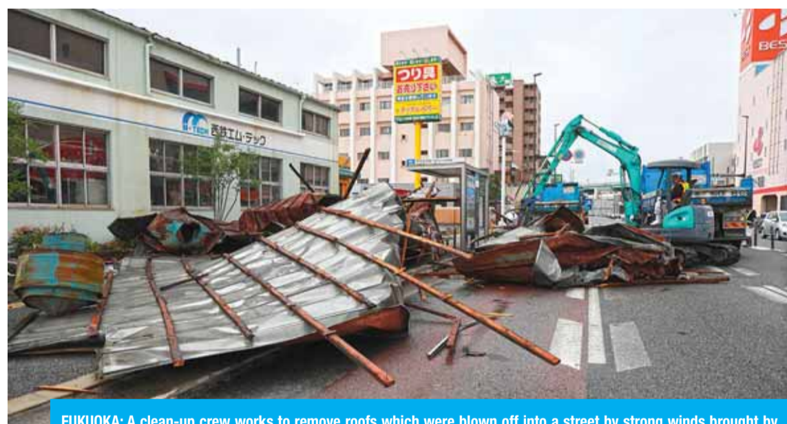
FUKUOKA: A clean-up crew works to remove roofs which were blown off into a street by strong winds brought by Typhoon Haishen in Fukuoka as the storm passes the southern Japanese island of Kyushu yesterday. — AFP
