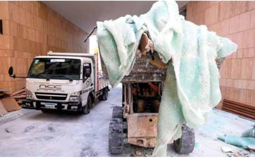
A construction vehicle clears glass from a damaged building in Beirut's Gemmayzeh neighborhood.
