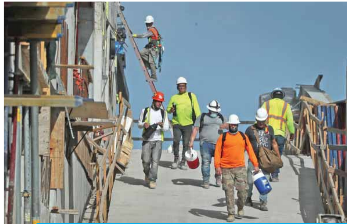
MIAMI, Florida: Construction workers are seen on a job site on Friday in Miami, Florida. The Bureau of Labor Statistics released a report Friday that shows the unemployment rate fell to 8.4 percent last month, down from a COVID-19 pandemic peak of 14.7 percent in April. — AFP
