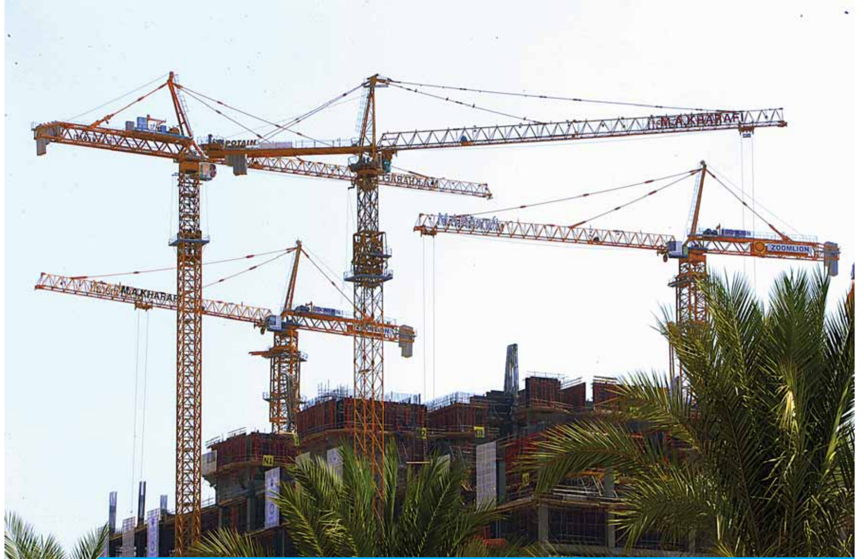
KUWAIT: Tower cranes at a major government construction project in Kuwait City. —Photo by Yasser Al-Zayyat
