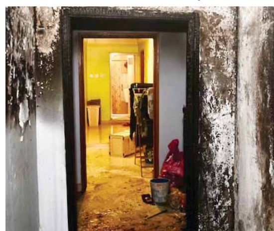
The scene inside the Ardiya house after the fire was extinguished.
