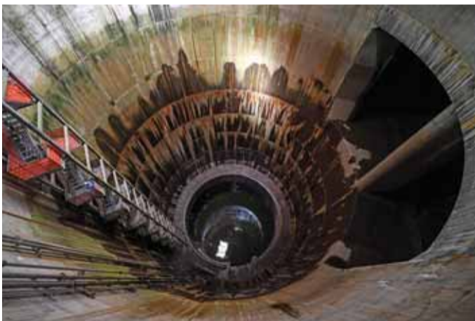
The 72.1 meter-deep number 1 tank of the metropolitan outer underground discharge channel is seen in Kasukabe.
