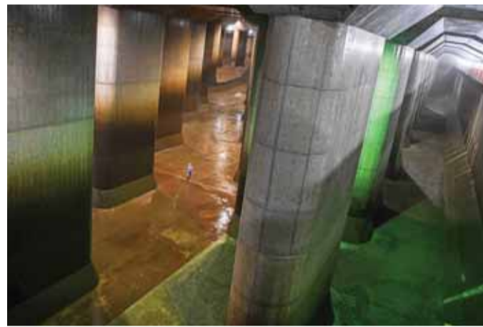
An employee walks in the water tank of the metropolitan. — AFP photos
