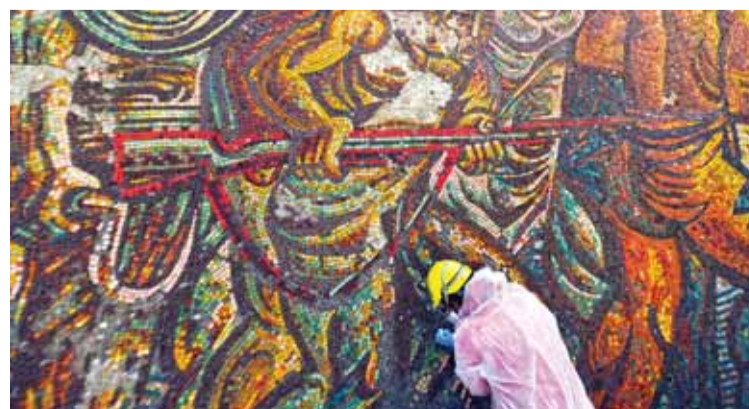
A construction expert works on a mosaic inside the House of the Bulgarian Communist Party on Buzludzha peak in central Bulgaria.
