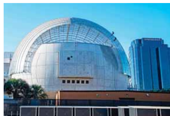
In this file photo workers clean the roof of the new Academy Museum of Motion Pictures, in Los Angeles, California.
