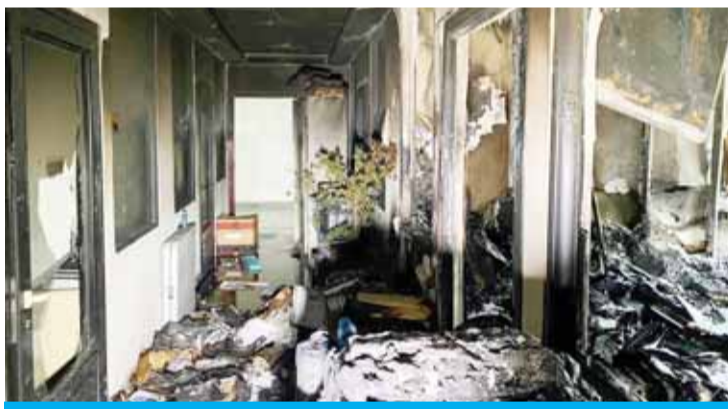
KUWAIT: Heavy damage left by a fire at an office in the Health Ministry building yesterday.
