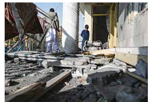
KABUL: People inspect a damaged house after several rockets land at Khair Khana, north west of Kabul yesterday. —AFP
