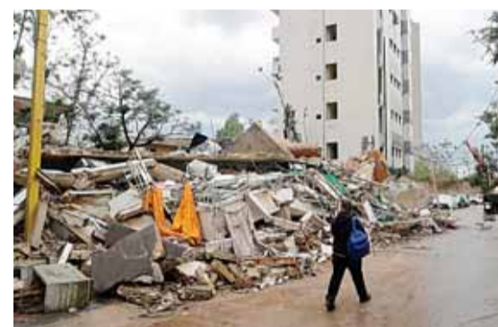
BEIRUT: A man walks past a building damaged by the August 4 port blast that collapsed due to heavy rain in the Karantina neighborhood on Nov 5, 2020. —AFP
