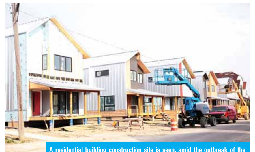
A residential building construction site is seen, amid the outbreak of the coronavirus disease (COVID-19), in Detroit, Michigan.—Reuters
