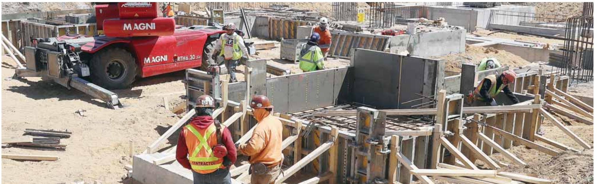
OCEANSIDE, New York: Construction workers perform their jobs in front of Mount Sinai South Nassau Hospital in Oceanside, New York. —AFP
