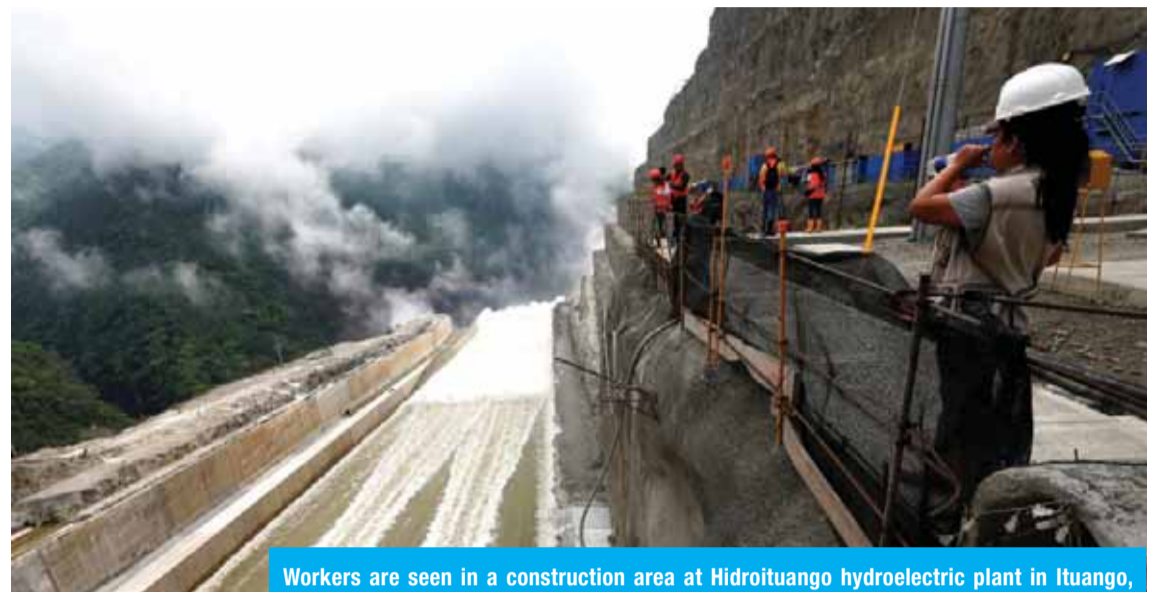
Workers are seen in a construction area at Hidroituango hydroelectric plant in Ituango, Colombia.— Reuters
