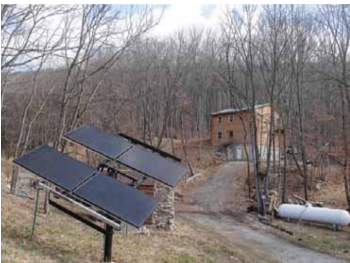
Solar panels are seen at the Fortitude Ranch in Mathias.
