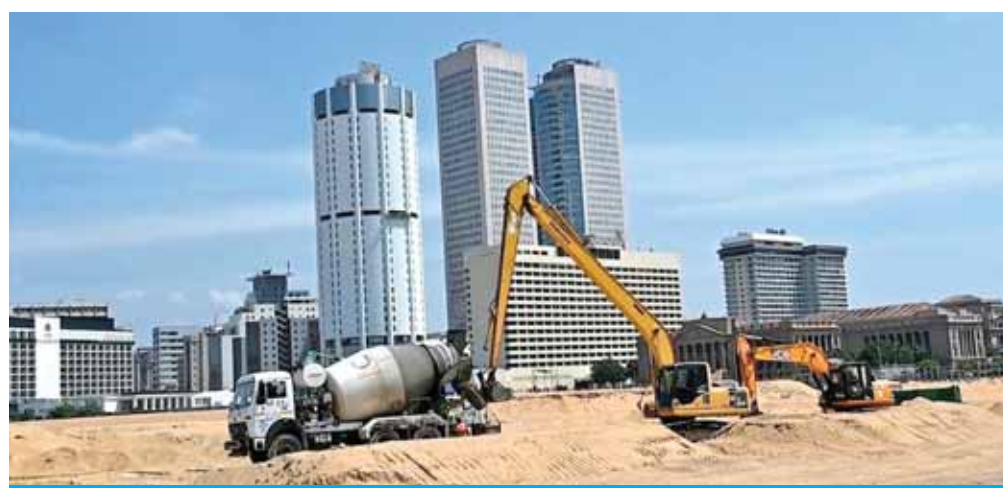
At Colombo's Port City — an artificial island the size of central London that is to house one of South Asia's biggest financial centres — work is progress. — AFP
