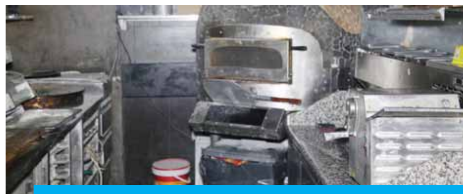
Damage left by a fire reported inside a Sulaibikhat supermarket's restaurant.
