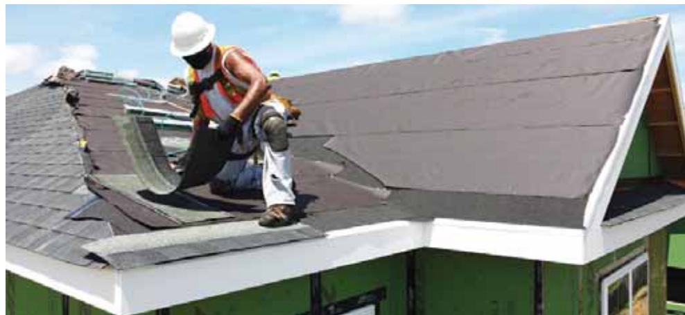
NEW YORK: In this file photo an aerial view is seen of a construction worker roofing an apartment home in Uniondale, New York. New home construction in May rose 4.3 percent compared to April, the Commerce Department said.—AFP
