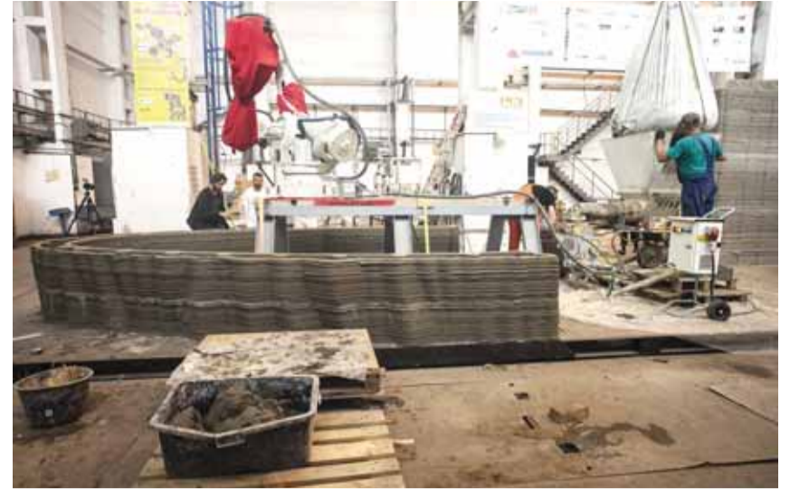
Workers check the 3D printing of the first-ever concrete house in Czech Republic.
