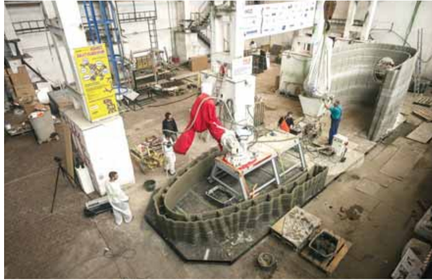
Workers check the 3D printing of the first-ever concrete house in Czech Republic.
