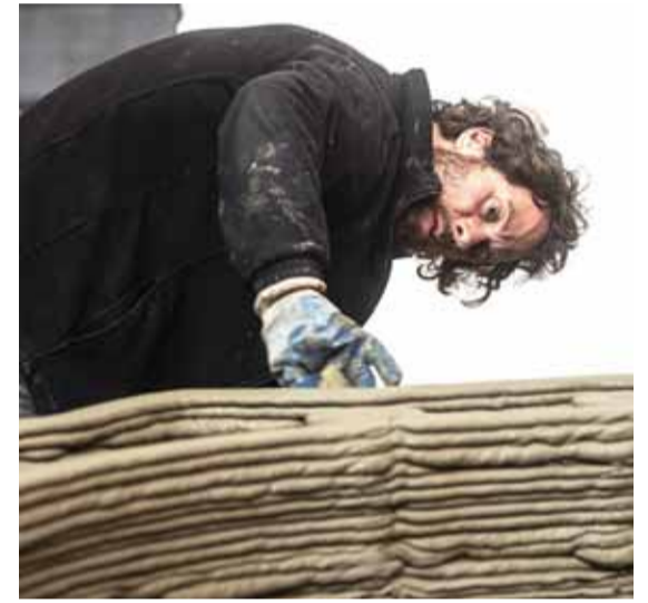
Sculptor Michal Trpak checks the 3D printing of first-ever concrete house in Czech Republic.
