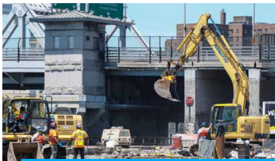
NEW YORK: Construction workers return to their jobs as part of phase one of reopening of the city from the coronavirus lockdown on Monday in the Bronx borough of New York City. — AFP
