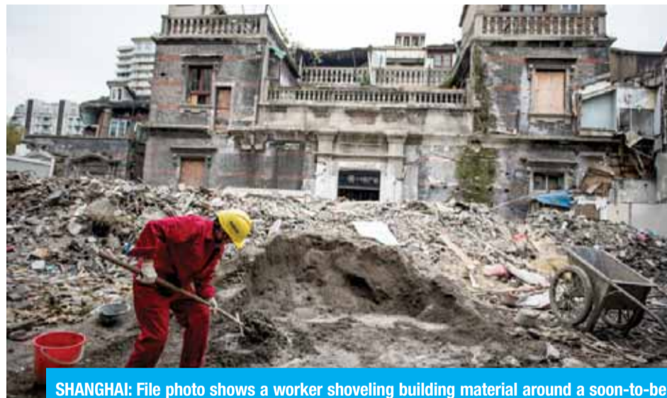
SHANGHAI: File photo shows a worker shoveling building material around a soon-to-be torn down and empty residential building in Shanghai. — AFP
