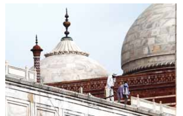
In this picture taken on Sunday, workers stand on the railing of the Taj Mahal after it was damaged due to heavy rainstorm in Agra.—AFP
