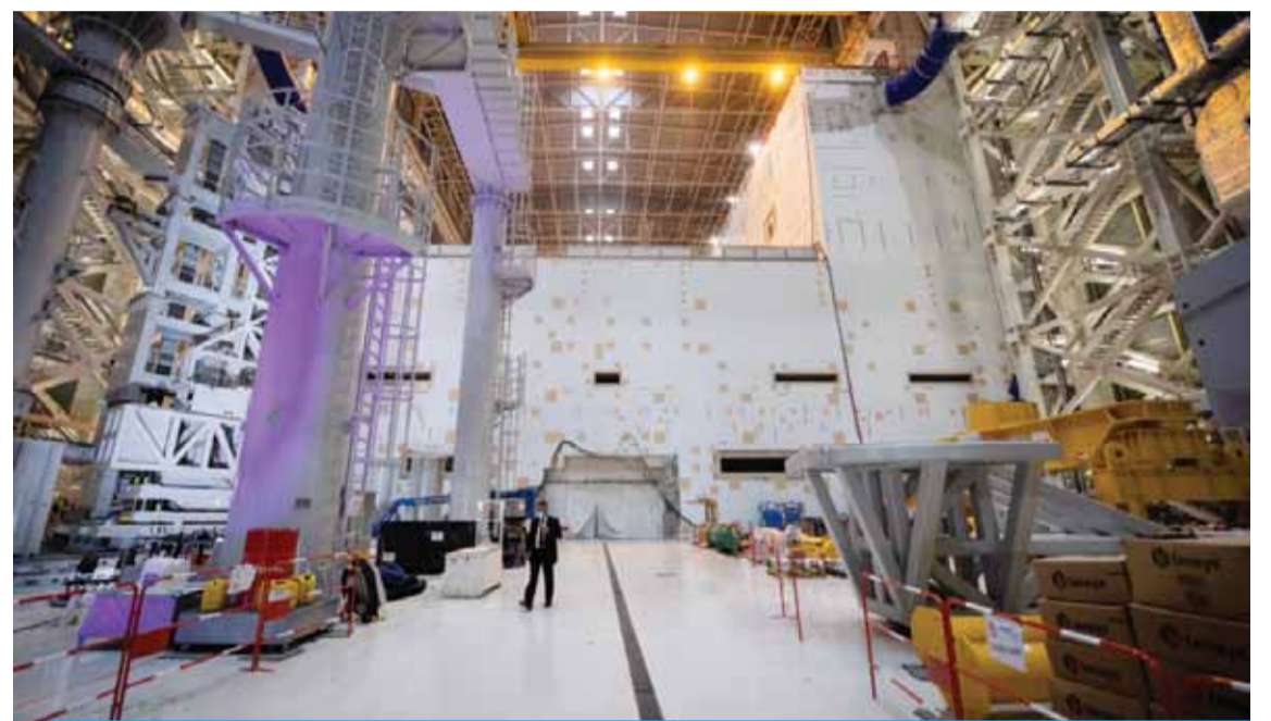
A picture shows the exterior of the Tokamak seen from the assembly hall during the launch of the assembly stage of nuclear fusion machine "Tokamak" of the International Thermonuclear Experimental Reactor (ITER) in Saint-Paul-les-Durance, southeastern France, on Tuesday.—AFP
