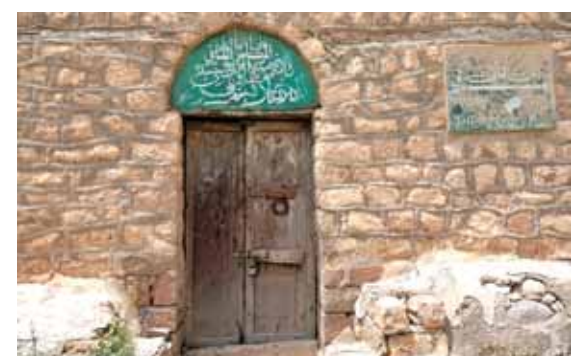
A picture shows a facade that is not destroyed at the National Museum.
