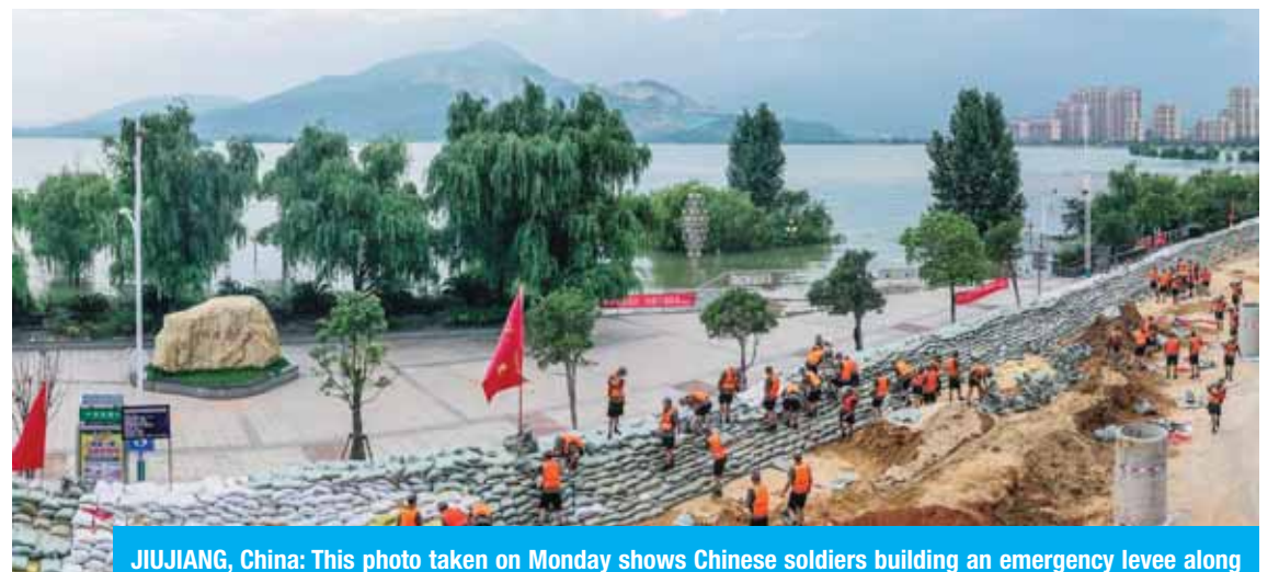
JIUJIANG, China: This photo taken on Monday shows Chinese soldiers building an emergency levee along the shore of Poyang lake to contain flooding due to seasonal rains and the swollen Yangtze River. — AFP
