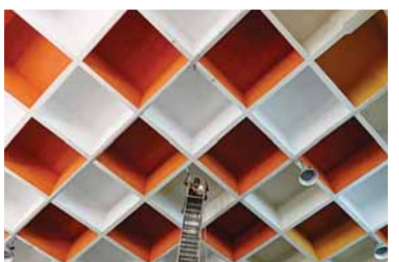
CHENNAI: A worker paints the ceiling of MGR central railway station in Chennai. India has opened up its vast railway sector to private companies, allowing firms to operate trains on certain routes, in a bid to boost its stuttering, virus-hit economy. —AFP
