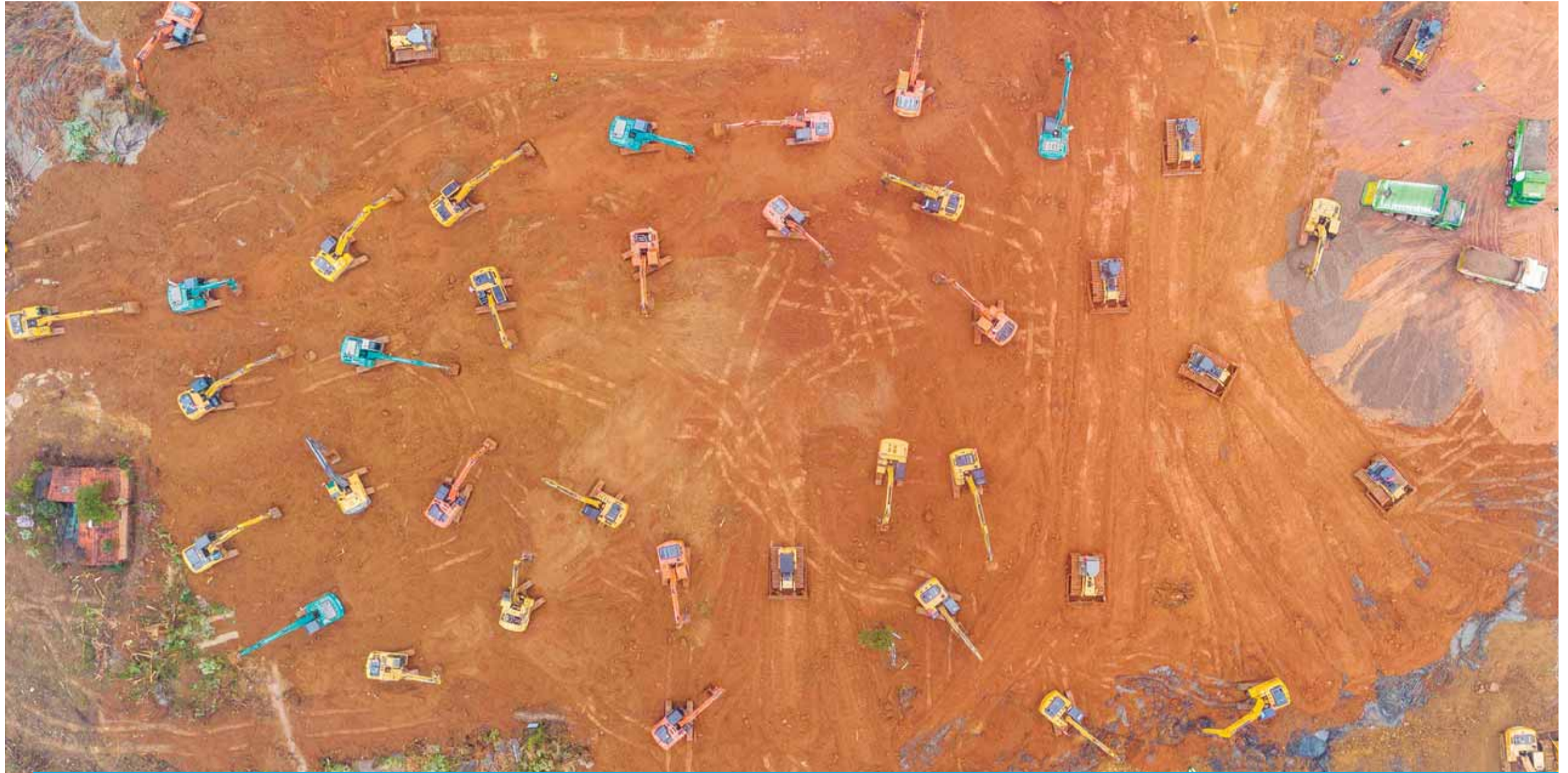
This aerial Friday photo shows excavators at the construction site of a new hospital being built to treat patients from a deadly virus outbreak in Wuhan in China's central Hubei province. — AFP
