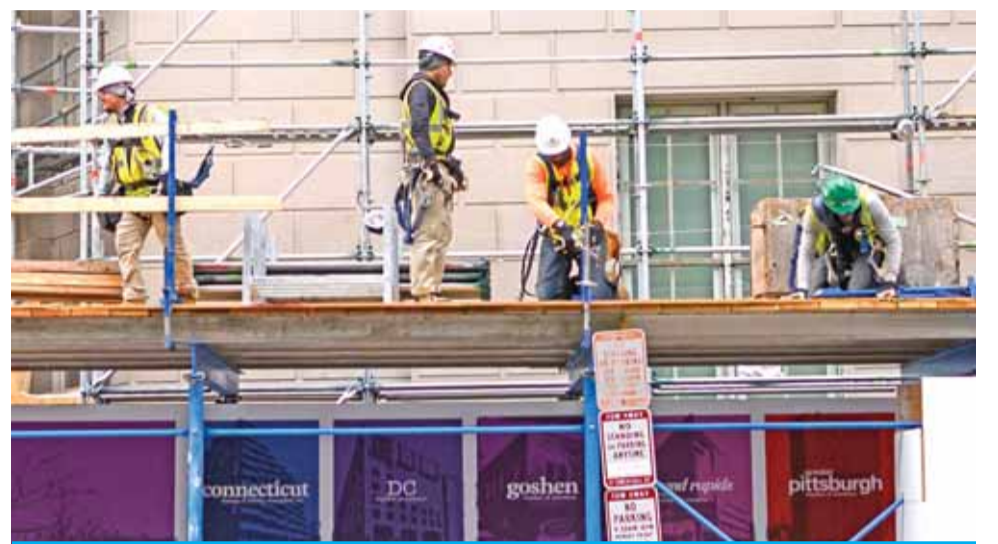
WASHINGTON, DC: In this file photo, construction workers put up support scaffolding on the side of a building in Washington, DC. America's solid job creation continued in December but at a slower pace while wages cooled off, according to the closely-watched government report released on Friday. — AFP
