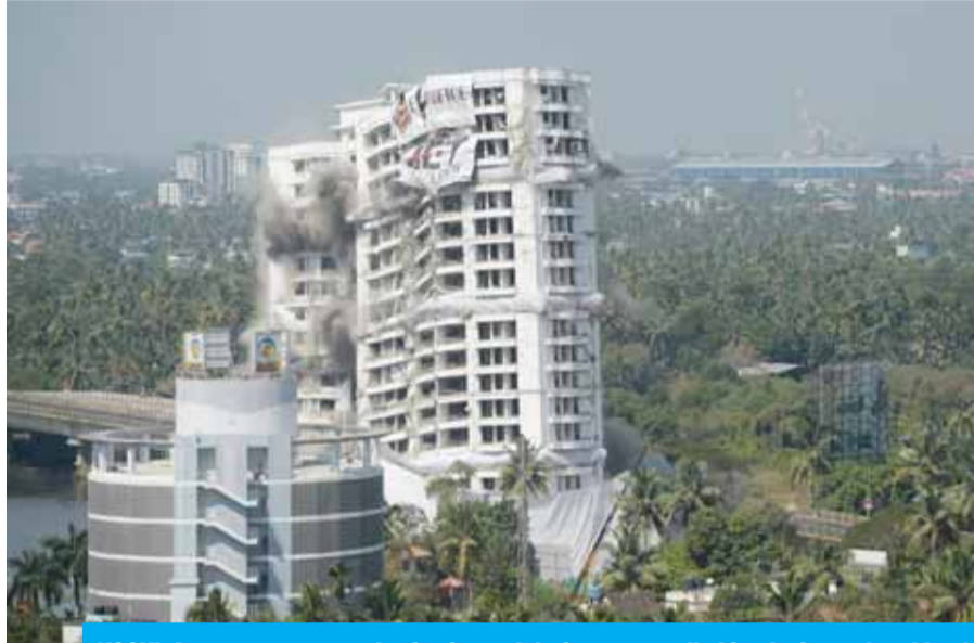
KOCHI: An apartment complex is pictured during a controlled implosion ordered by the Supreme Court for violating coastal construction regulations in Kochi yesterday. — AFP
