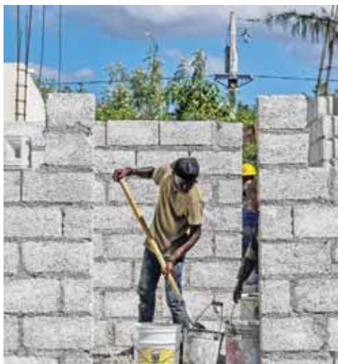
A laborer works at a construction site in Croix des Bouquets on December 30, 2019
