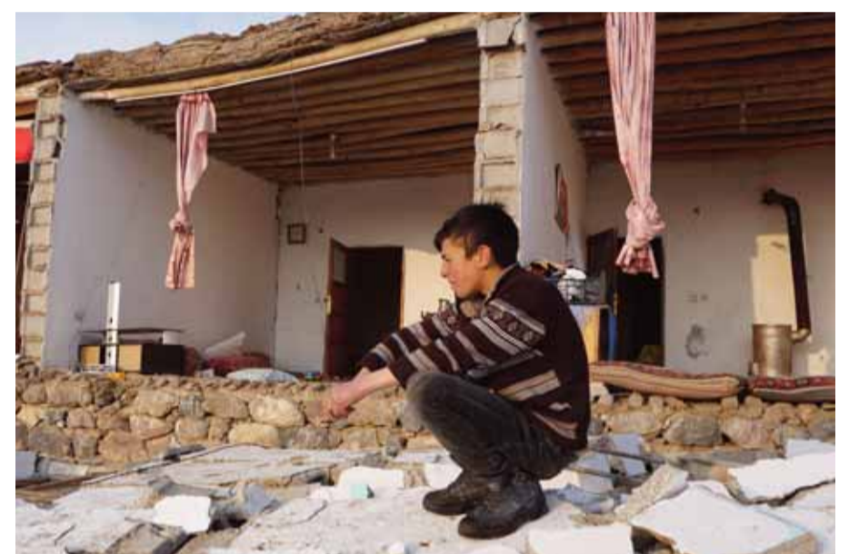
BASKALE, Turkey: A Turkish child kneels by a destroyed house in Van province after an earthquake struck northwestern Iran yesterday. — AFP
