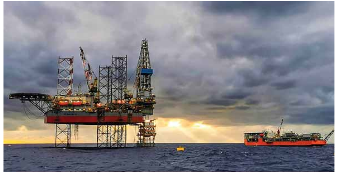
This undated handout photo released by Cambodia's Ministry of Mines and Energy shows an offshore oil platform under construction off the Cambodian coast.—AFP
