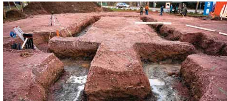
View of the ground laying work in the center of Stiege for the Stabkirche.
