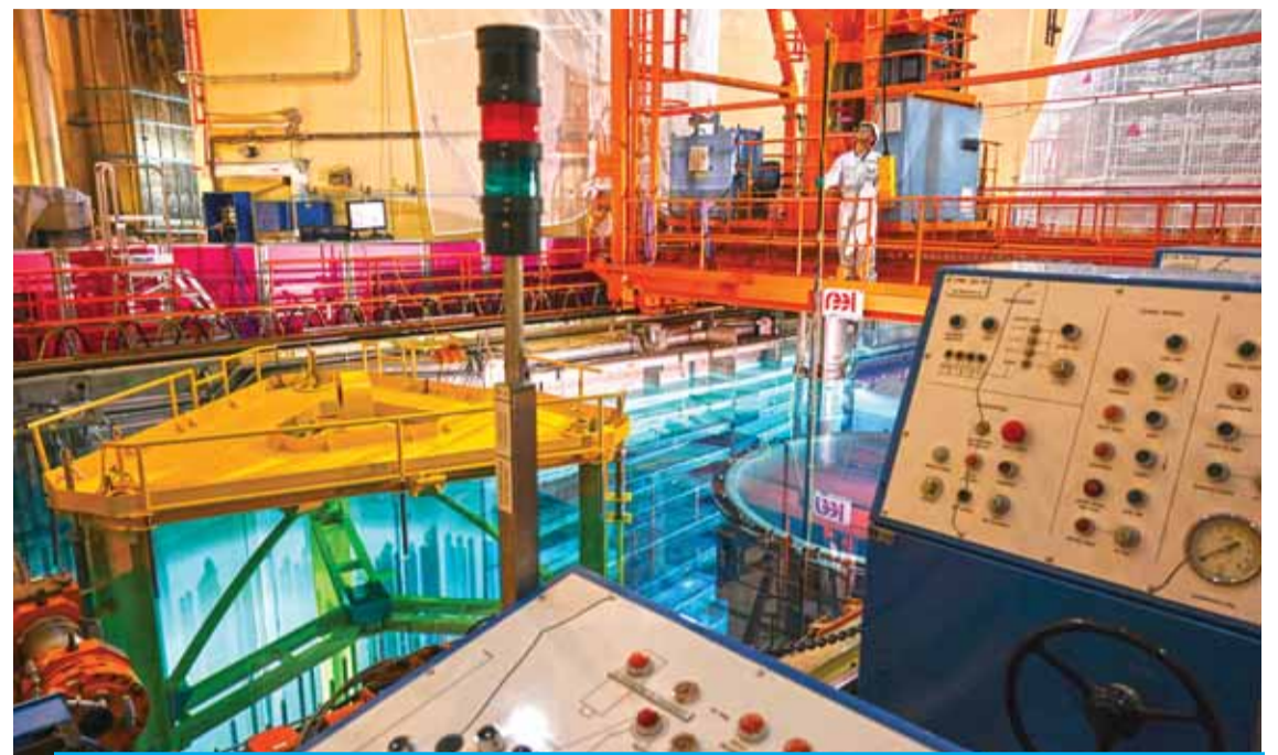
In this file photo taken on June 27, 2019, a man works in the hearth of the nuclear reactor building at the Tricastin nuclear power plant owned and operated by French energy company EDF in Saint-Paul-Trois-Châteaux, southern France. — AFP
