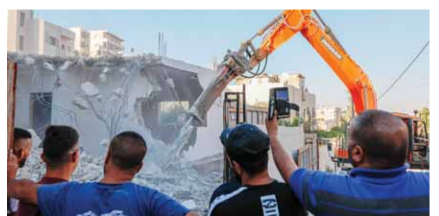
JERUSALEM: Relatives of the Palestinian Shalalda family watch as an excavator hired by them demolishes their family home in Al-Tur on July 2, 2020. — AFP
