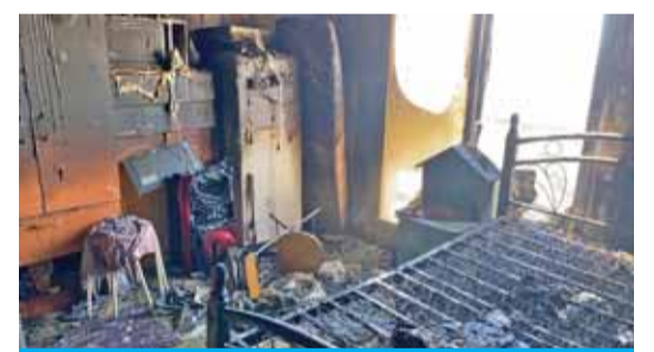
Heavy damage left by a fire reported in a Farwaniya apartment.
