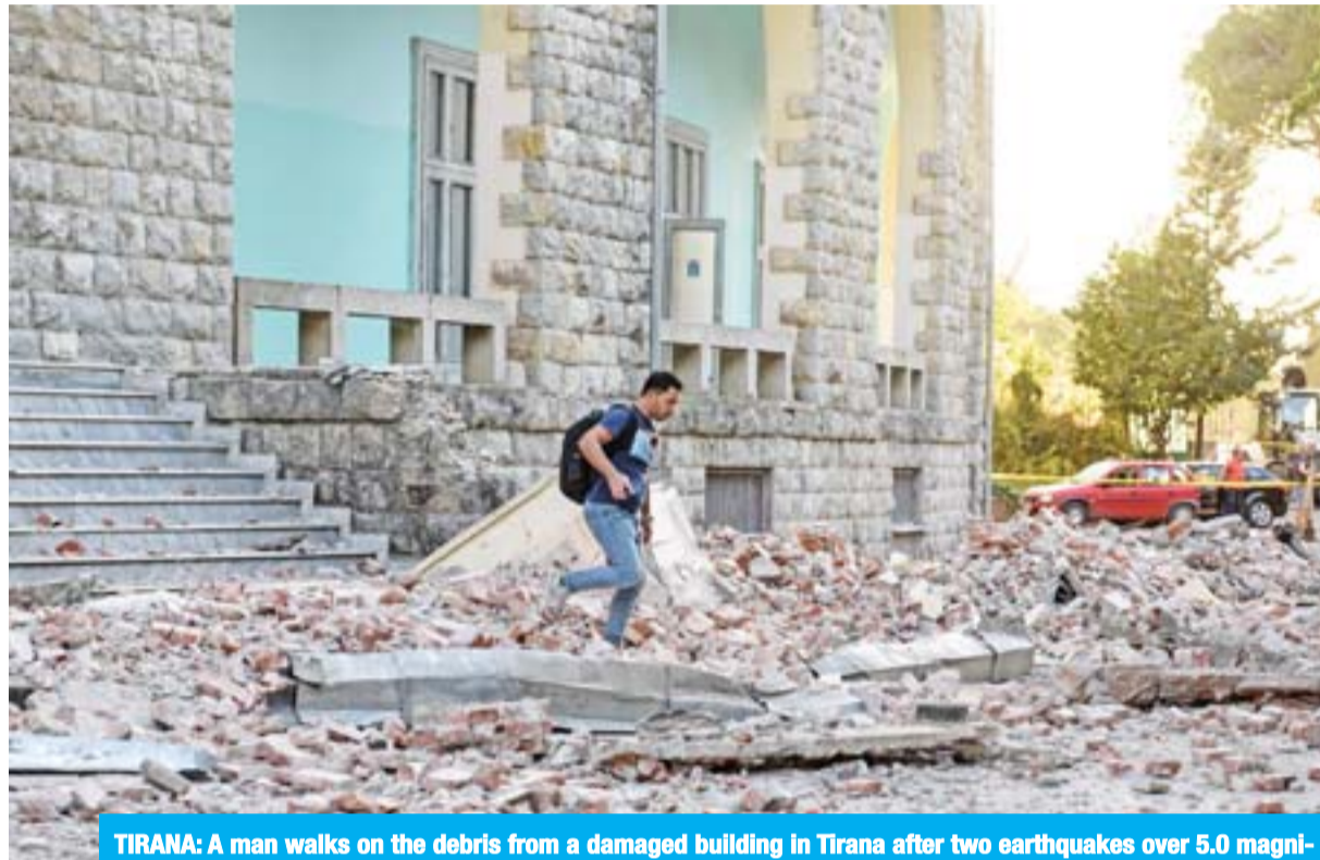
TIRANA: A man walks on the debris from a damaged building in Tirana after two earthquakes over 5.0 magnitude struck the coastline Adriatic coastline of Albania. — AFP
