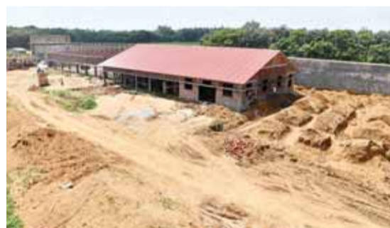
ASSAM: Photo shows an under-construction detention centre for people who are not included in a 'citizens register' in Kadamtola Gopalpur village, in Goalpara district. — AFP
