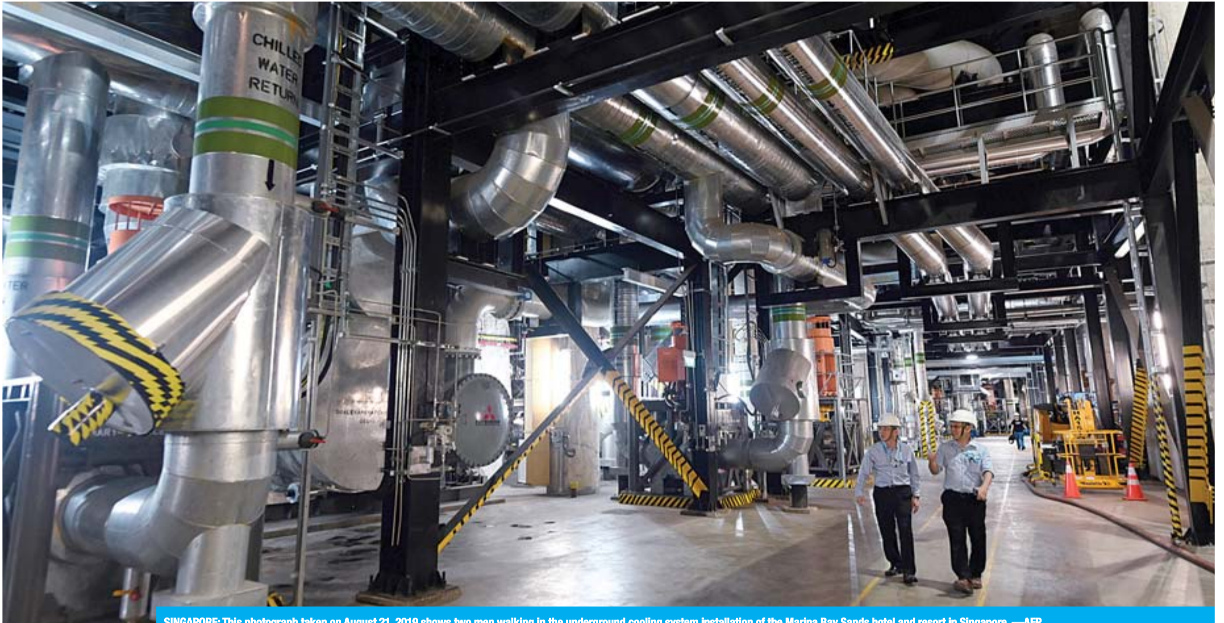
SINGAPORE: This photograph taken on August 21, 2019 shows two men walking in the underground cooling system installation of the Marina Bay Sands hotel and resort in Singapore. —AFP
