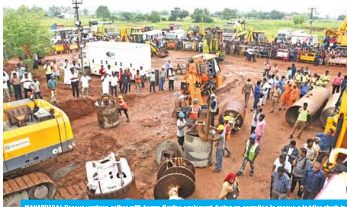
MANAPPARAL: Rescue workers gather with heavy digging equipment during an operation to rescue a toddler stuck in a deep well near Manapparal town in Tiruchirappalli district, in India's southern Tamil Nadu state yesterday. — AFP
