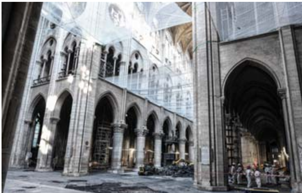
This file photo shows damage on the nave and rubble during preliminary work in the Notre-Dame de Paris Cathedral three months after a major fire.
