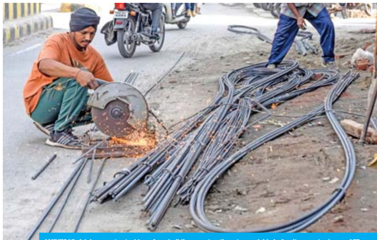
AMRITSAR: A laborer cuts steel bars for a building construction at a roadside in Amritsar yesterday. — AFP
